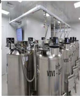
Pathogens Biobank IPK Liquid Nitrogen freezer room
